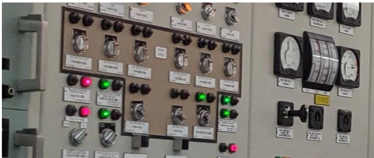
Nuclear Plant Control Room Switches and Components
